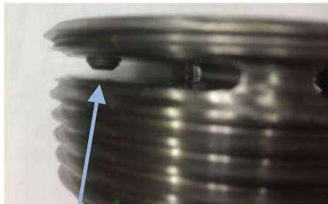
Partially Loose Set screw
