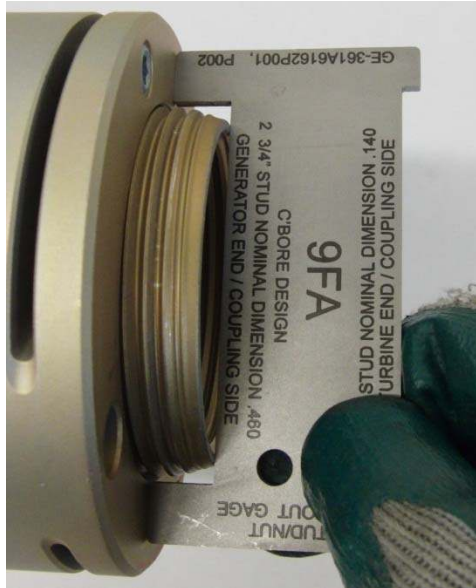
Picture 6C – Use of Stick-Out Gage on Load Coupling or Steam Turbine to Generator Bolted Flange Connection
