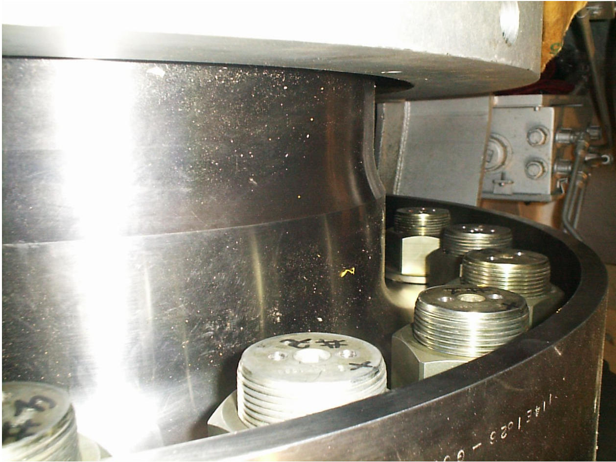
Photo 2 Back Side of 9FA turbine flange showing studs and nuts in place
