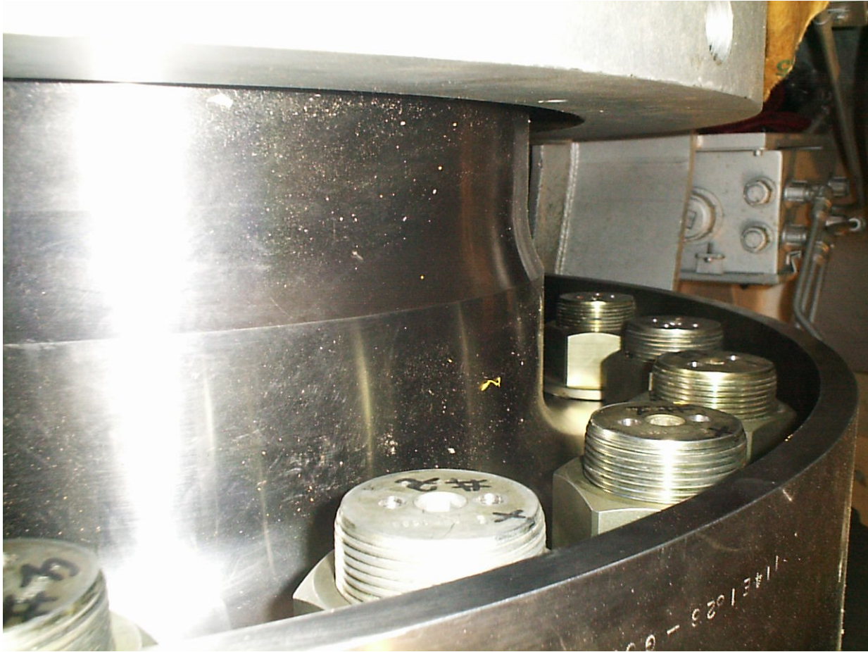
Photo 2 Back Side of 9FA turbine flange showing studs and nuts in place
