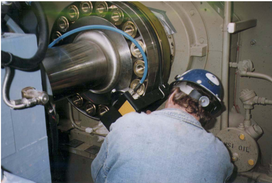
Photo 4 View of 1-1/8" puller tool and safety cage mounted on turbine to coupling flange of 6FA machine. Tool is pressurized and millwright is tightening nut.
